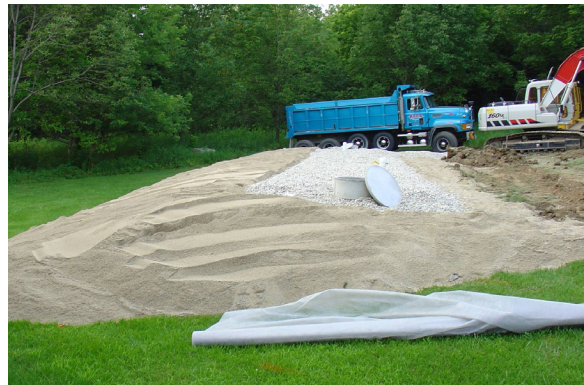
There are several different types of POWTS including at-grade, conventional systems, constructed-wetland, dripline, in-ground pressure, mound systems, and holding tank systems. A mound system is pictured here.
